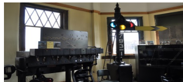
Controls-Model Boards & Signal.
